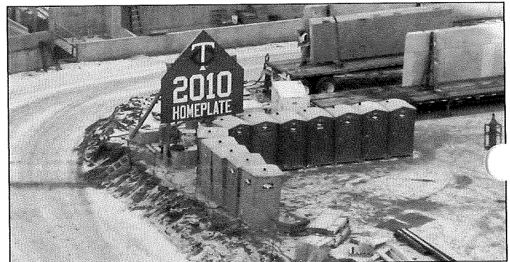
Dirt, mud, machinery, scaffolding, and portable toilets may have taken up temporary residence in the playing field of the new Twins Ballpark, but home plate will permanently remain. In about one year the Minnesota Twins will move in to their new location and begin the 2010 baseball season. Photo by Richard Kentzelman.
