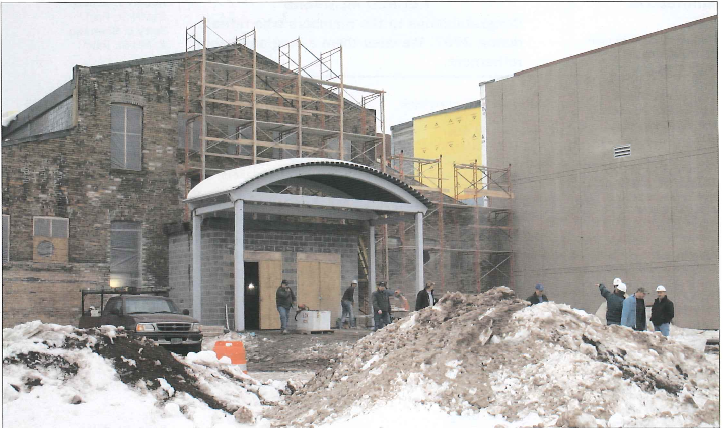
An exterior photo taken just before Christmas 2007 shows the original Clyde Iron, left, being converted to Heritage Hall, a central structure that will house concessions and utilities. To the right is the first of two sports pavilions.
