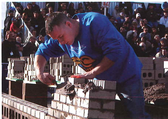
Patrick Baxter lays 13 bricks a minute on his way to being judged 'the world's best bricklayer.'
