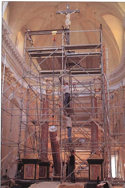
Prep work had included running steel cable through the column core, anchoring it at the bottom end and knotting the top end into an eyelet. With a hook through the eyelet, the men began working in unison to pull chain through a chainfall—the same procedure that's used to lift a grand piano. The column went up slowly, finally lifting into the air to be moved, suspended from a trolley on an I-beam, to center over its pedestal.
