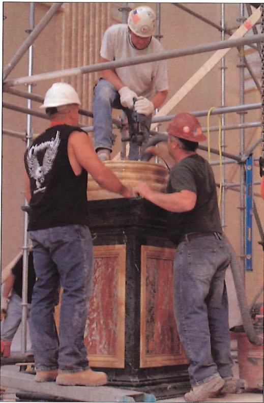
TCTM Foreman Curt Nelson drilled holes into the stone pedestal while Rob Frahm (left) and Ted Konz (right) assisted. Four half-inch stainless steel dowels were epoxied into the drilled holes. Mated with matching holes in the column base, the dowels provide alignment and keep the column from twisting or sliding.
