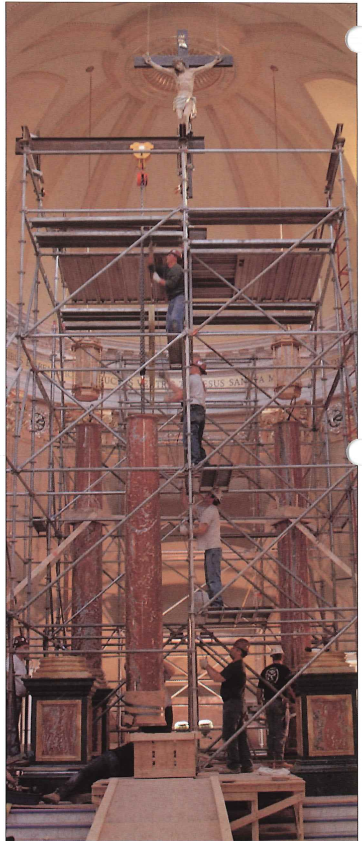
Four men on ascending scaffolding worked together to lift and place the third of four marble columns that ultimately will surround a marble tabernacle.
