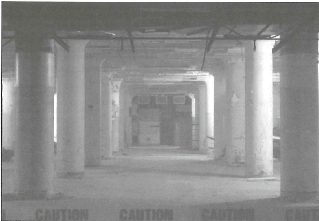
COLUMNS on 20-foot centers support the 17-story building. Peak construction is set during Spring 2005, when some 1,400 workers will be at the site, compared to about 300 working there last month. By the completion target date of May 31, 2006, an estimated $240 million will have been spent on the project.
