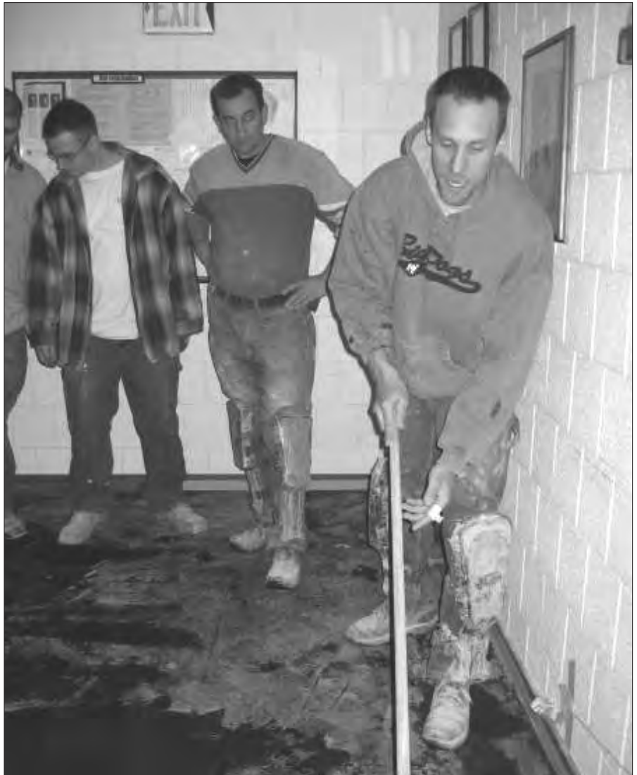
Apprentice Andrew Gunter applies the liquid membrane Fracture Guard 5000 while fellow apprentices Bodhi McKinney (left rear) and Jasmin Hurtic (right rear) watch.
